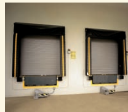
Rolling Service Doors
